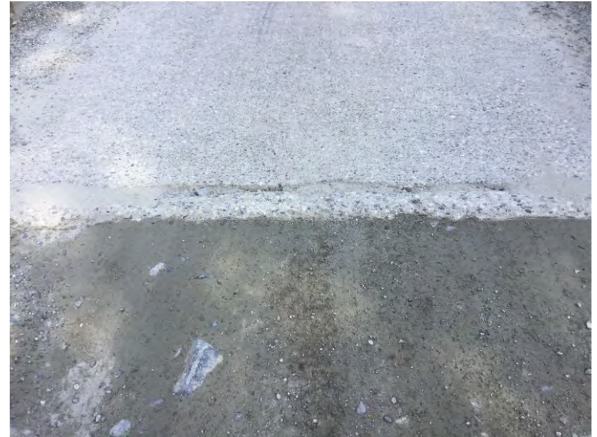
Minor wear damage noted to ballast wall and deck at right bank
