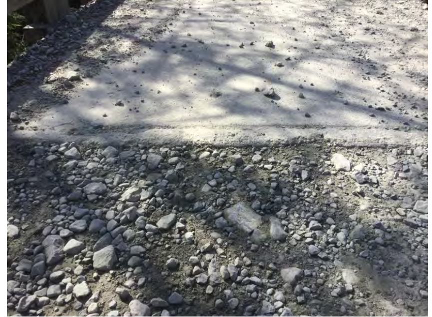
Minor wear damage noted to ballast wall and deck at left bank
